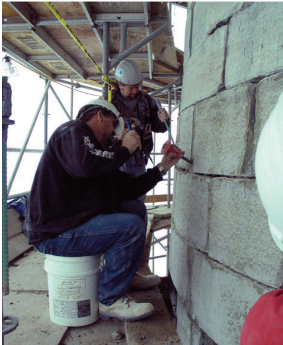
Workers removing deteriorated mortar from the East Branch ditch tower for repointing. Photo: © Fort Henry National Historic Site of Canada–Archives.
