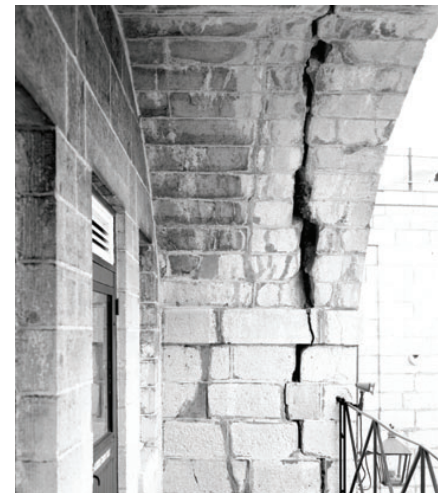
Fractures and spalling of the limestone blocks in an archway of the redoubt. The mortar joints had also deteriorated significantly. Photo: © Fort Henry National Historic Site of Canada–Archives.
