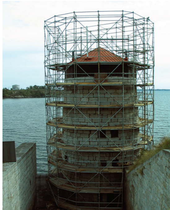
The scaffolded East Branch ditch tower during the restoration project. Photo: © Fort Henry National Historic Site of Canada–Archives.
