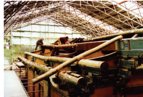
The Hall of Paradise, during restoration. Dismantlement of the temple allowed each building component to be documented individually. Photo: © Soon-Kwan Kim.
