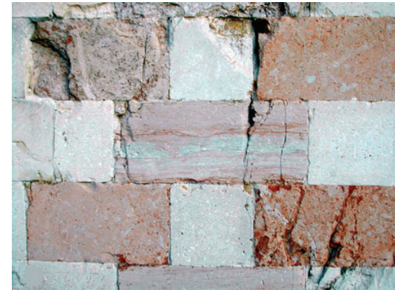
Detail showing the masonry deterioration of the facade caused by seismic stress. Photo: © Marco Tallini.
